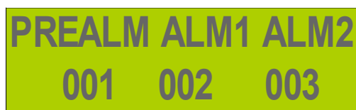
PROGRAMMED ALARM LEVELS
